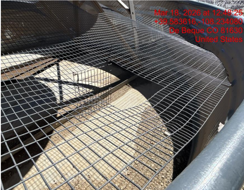
Wildlife Entry Hazard – Photo #03178
