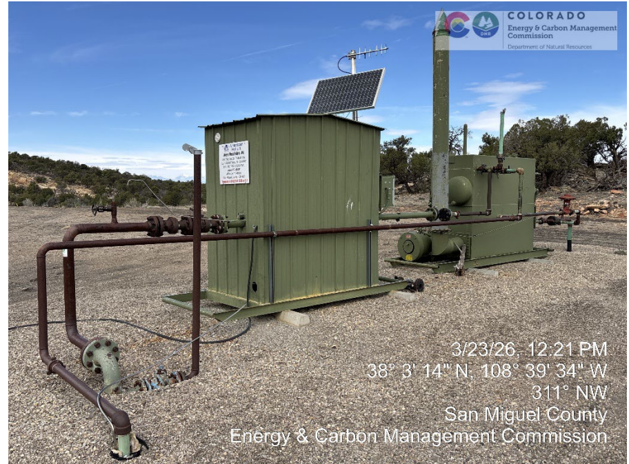
Separator and Meter housing with sign
