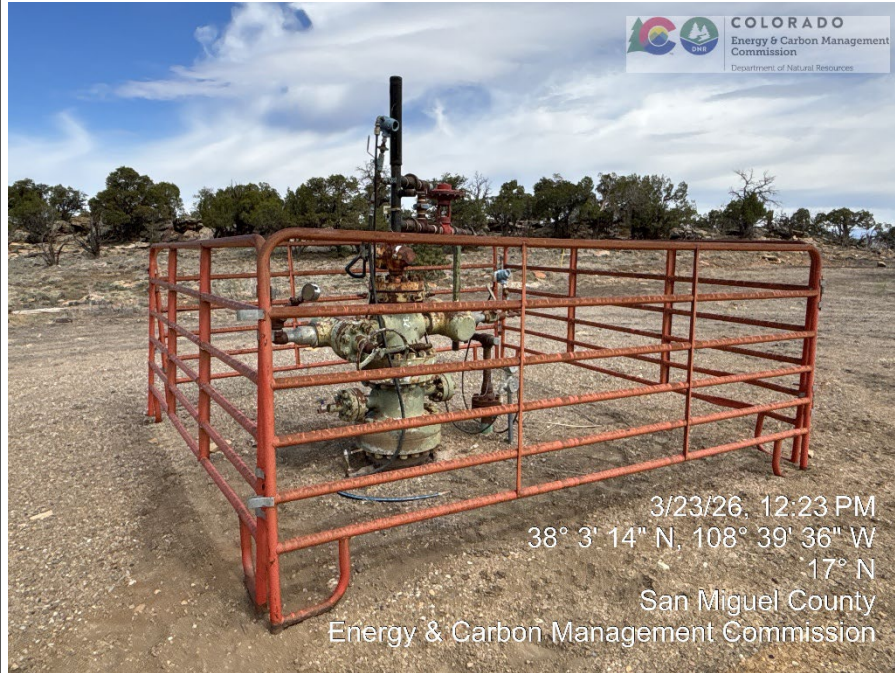
Wellhead with fence
