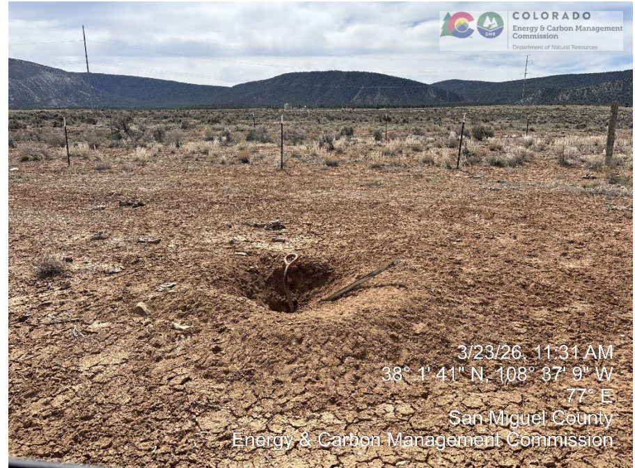
Unmarked guyline anchor
