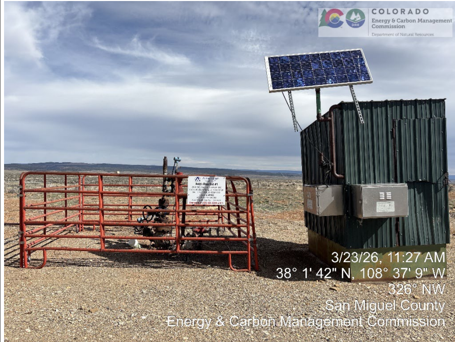
Wellhead with fence and sign
