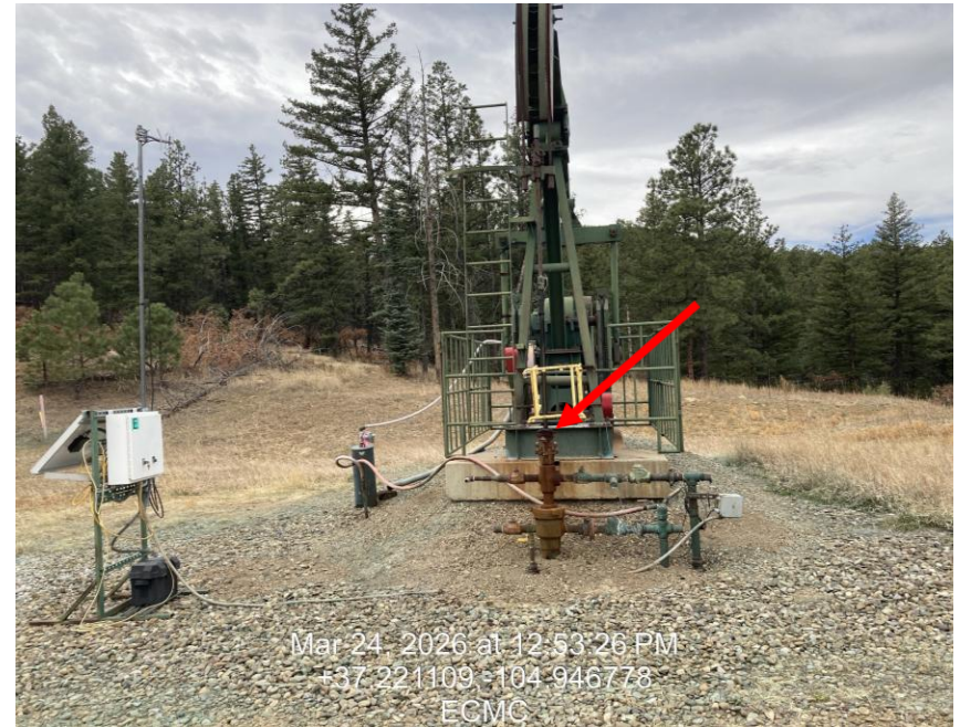
Photo 4: Original Wellhead and equipment, source of leak
