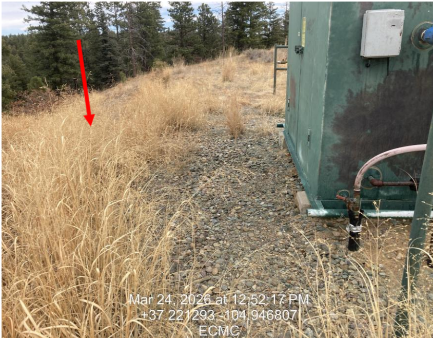
Photo 3: tall vegetation behind meter house
