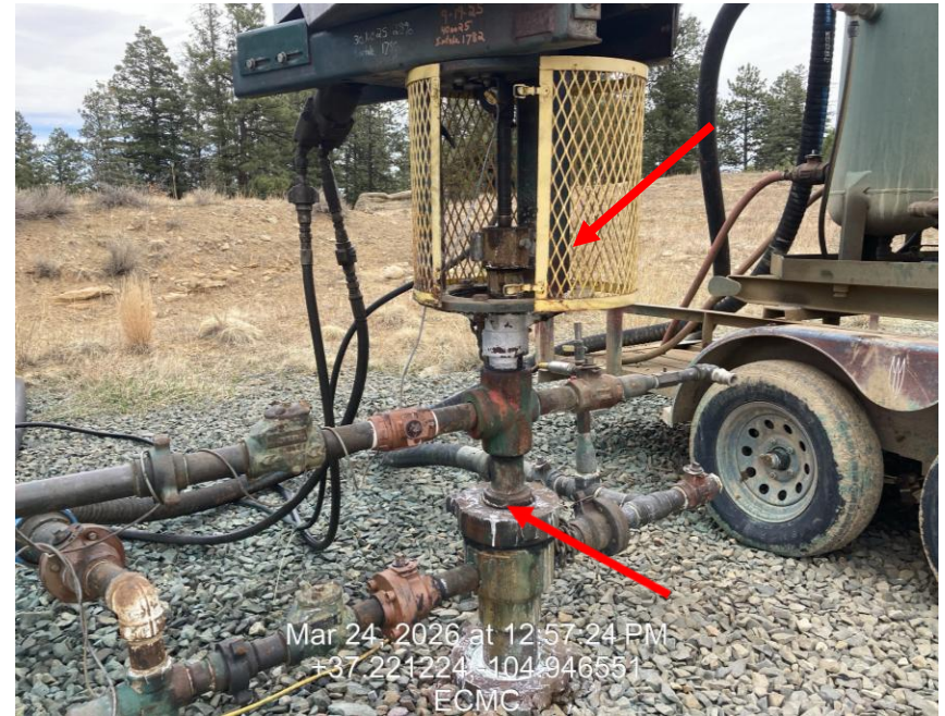
Photo 12: white staining on TR wellhead, standing water observed in pin-plate
