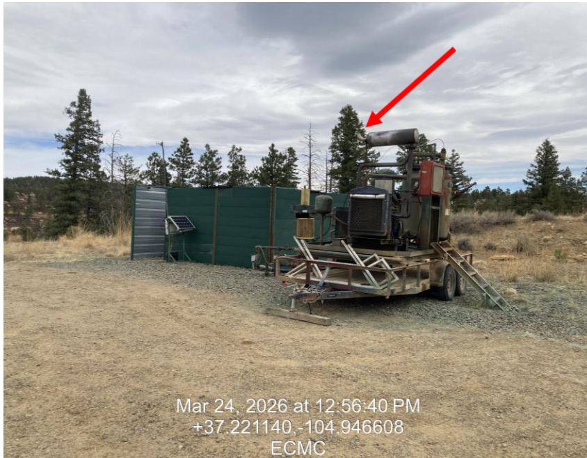
Photo 11: TR wellhead and equipment
