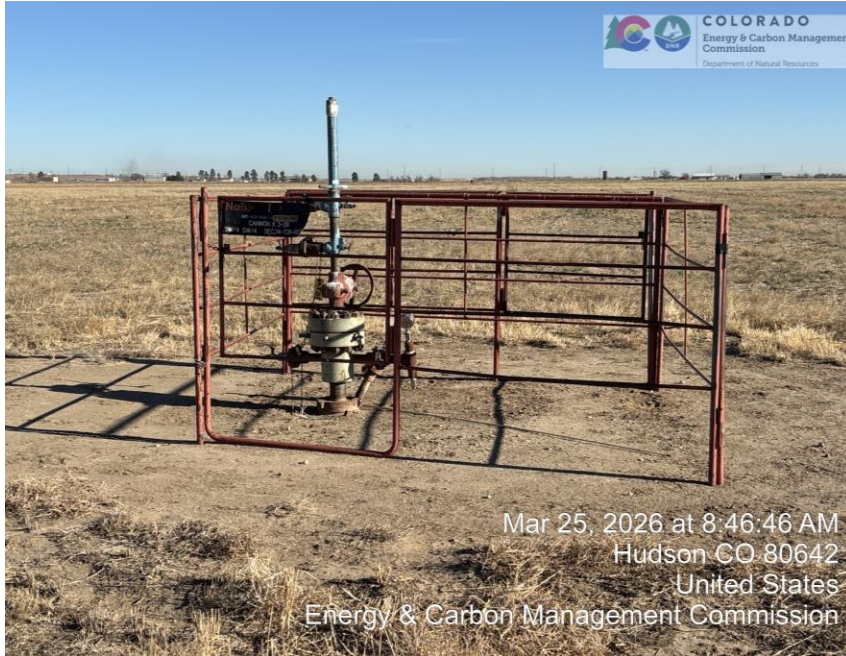
Photo 1 well head and equipment
