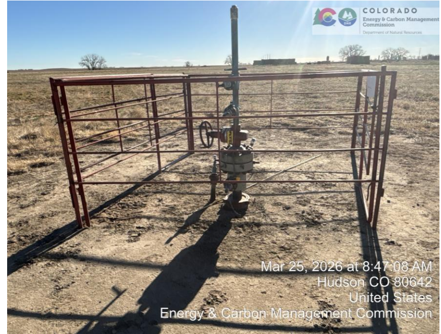
Photo 2 well head and equipment
