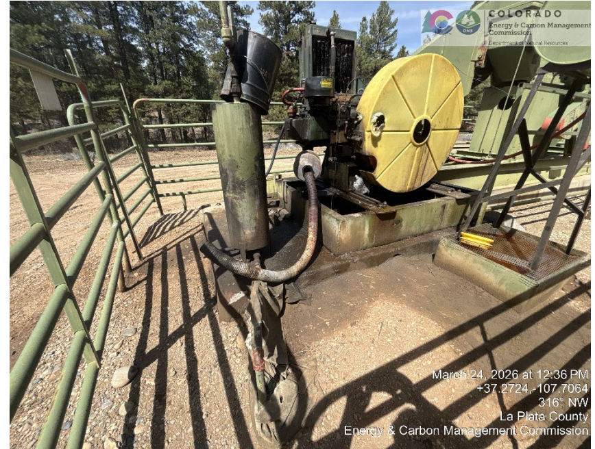
ENGINE OIL LEAK
