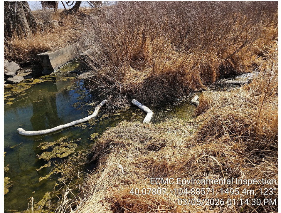
Photo 8 – Booms and mats placed in Big Dry Creek have not been maintained and are no longer effective in controlling the spread of impacts.
