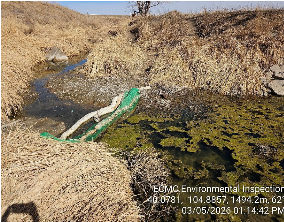
Photo 9 - Booms and mats placed in Big Dry Creek have not been maintained and require replacement.
