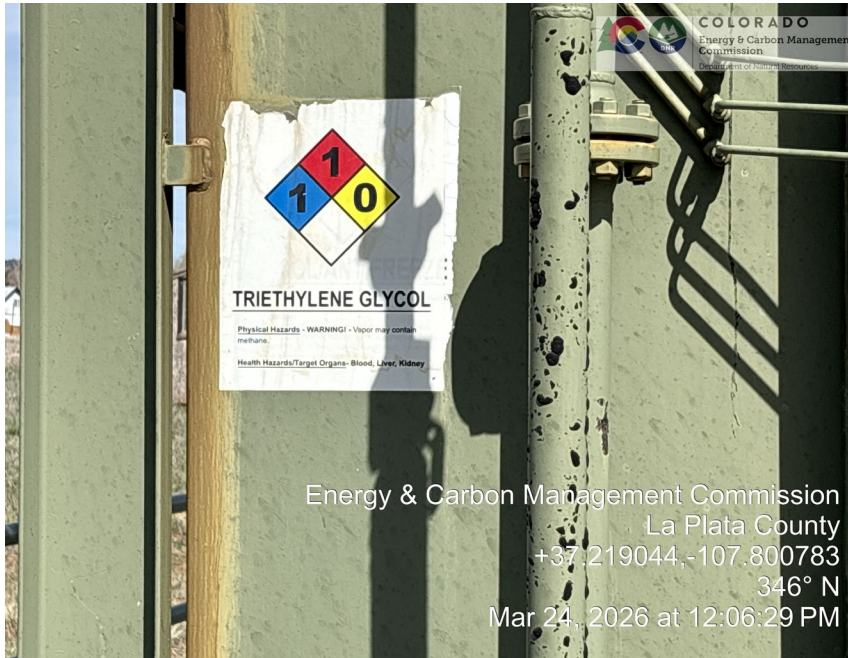
15. Hazcom placard on vertical heated separator.
