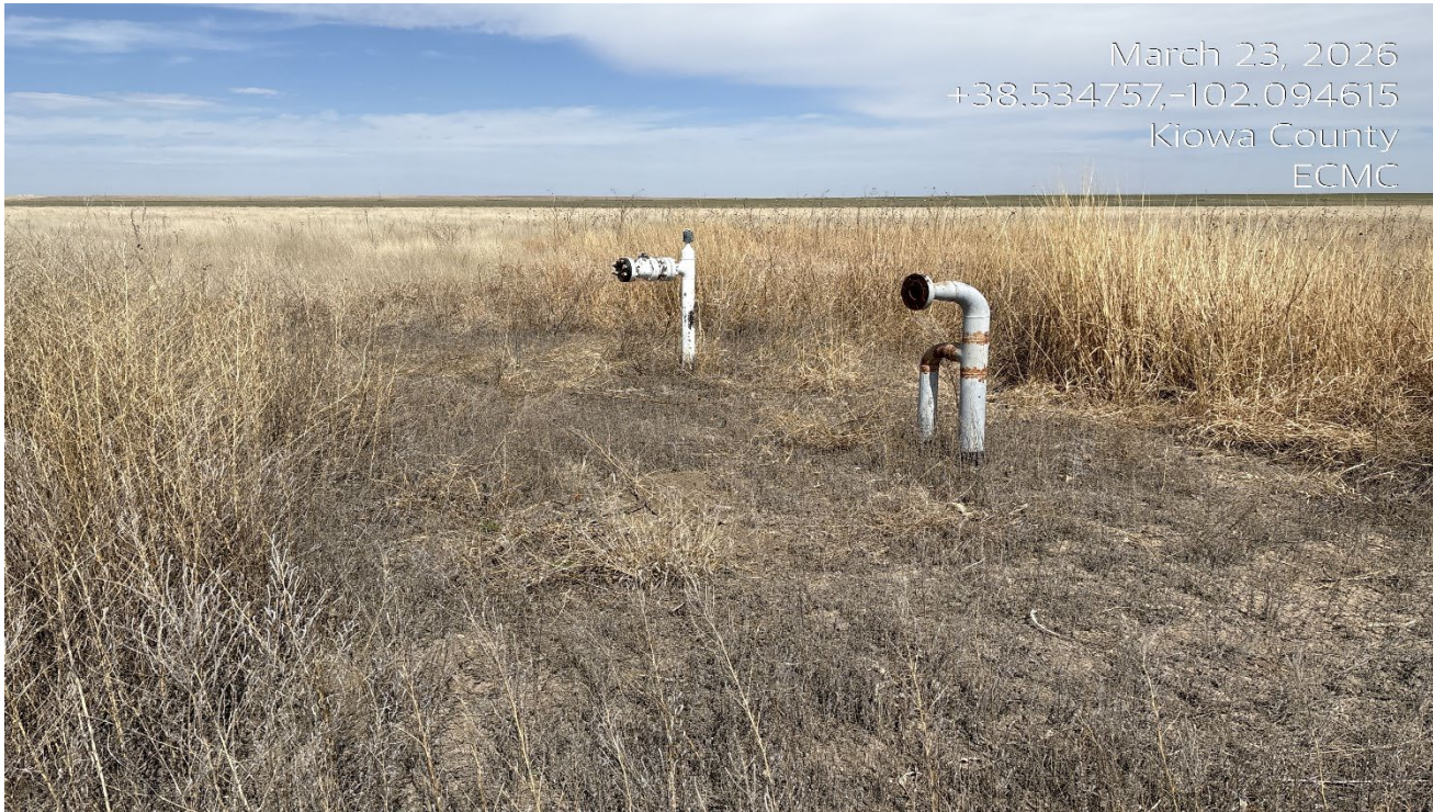
Photo 8. Facing toward the northeast side of the location. Abandoned pipe risers have not been removed.
