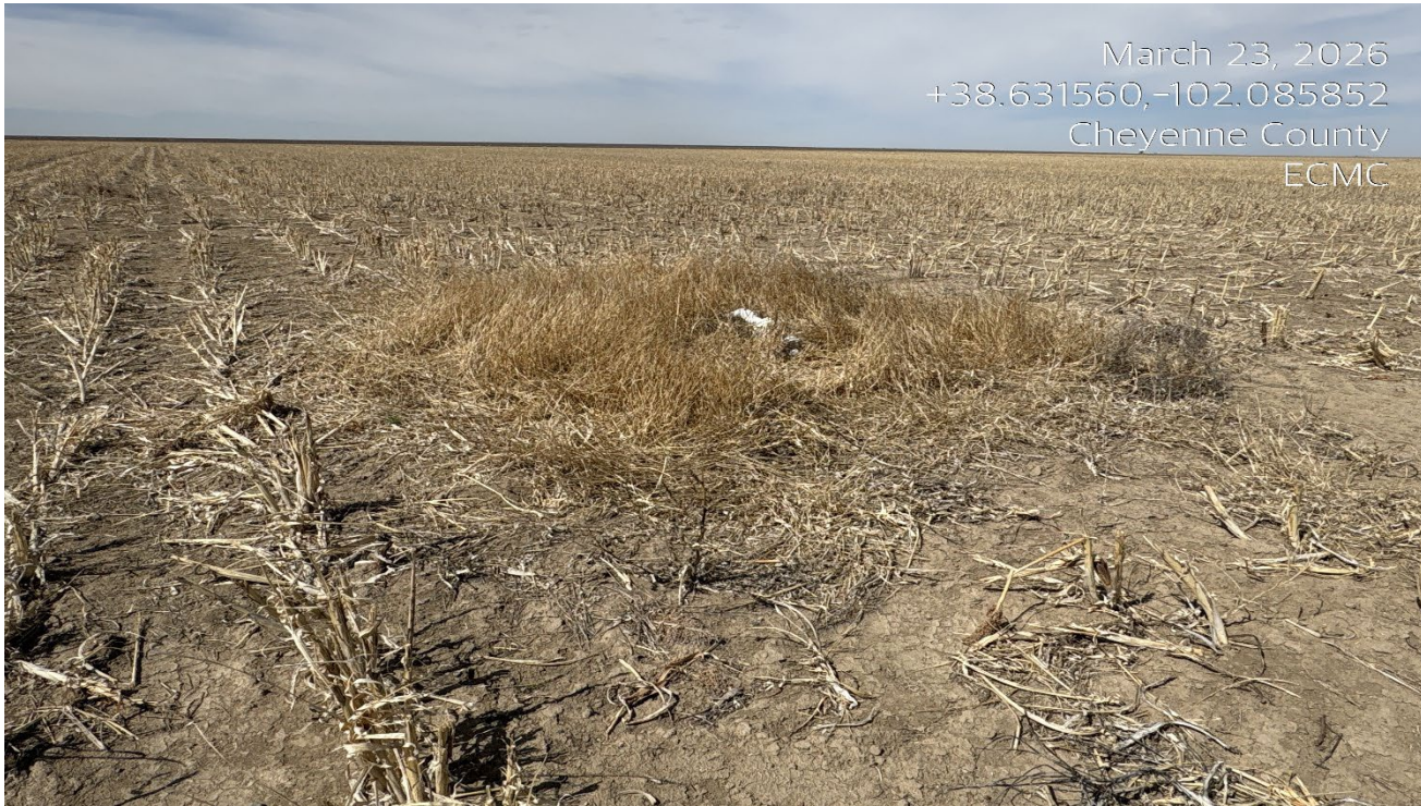
Photo 1. Facing west at the location. There is a pipe riser that needs to be removed. The riser is low to the ground and could be a farming hazard.
