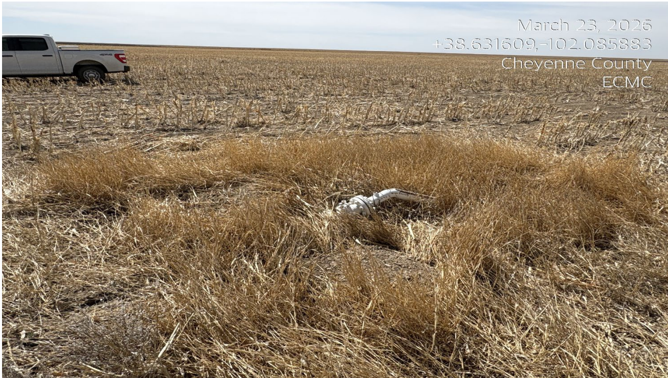
Photo 2. There is a pipe riser that needs to be removed. The riser is low to the ground and could be a farming hazard.
