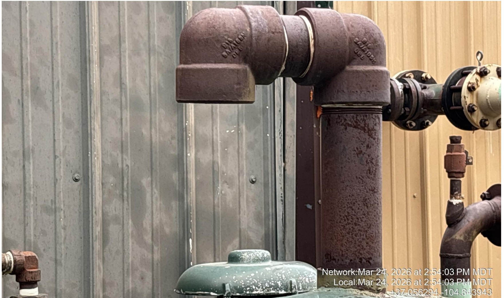
PHOTO 5: VENT ON PRODUCED WATER TANK DOES NOT HAVE WILDLIFE PROTECTION.
