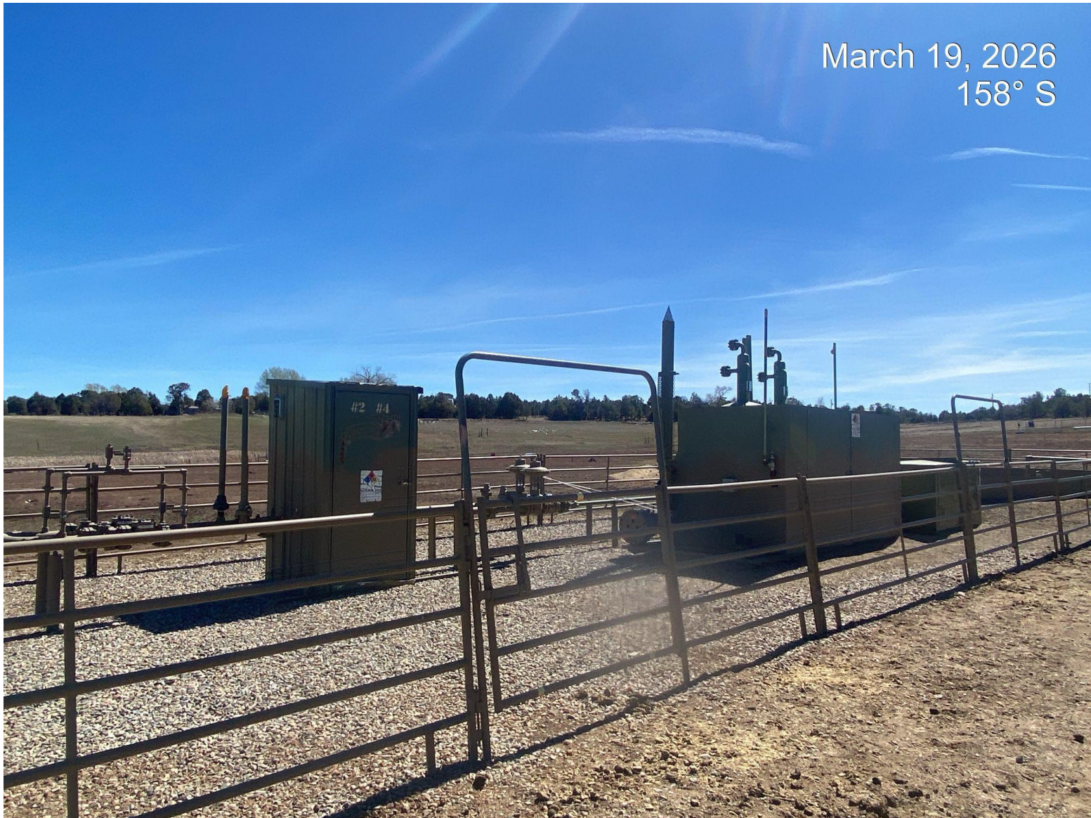
Photo 5. Labels at meter shed and separator equipment are starting to deteriorate.
