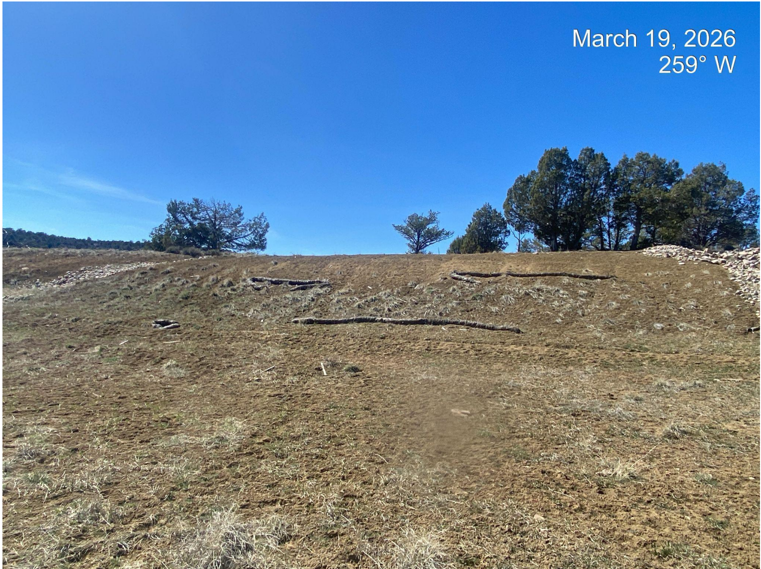
Photo 2. View of location cut slope with failing stormwater BMPs.
