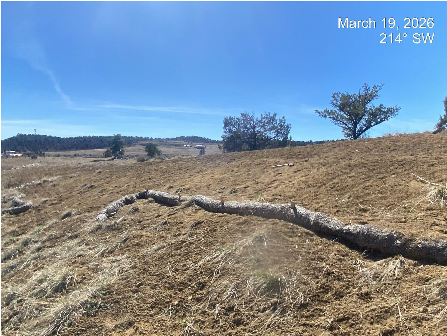
Photo 3. Failing stormwater BMPs that are not longer functioning on the location cut slope.
