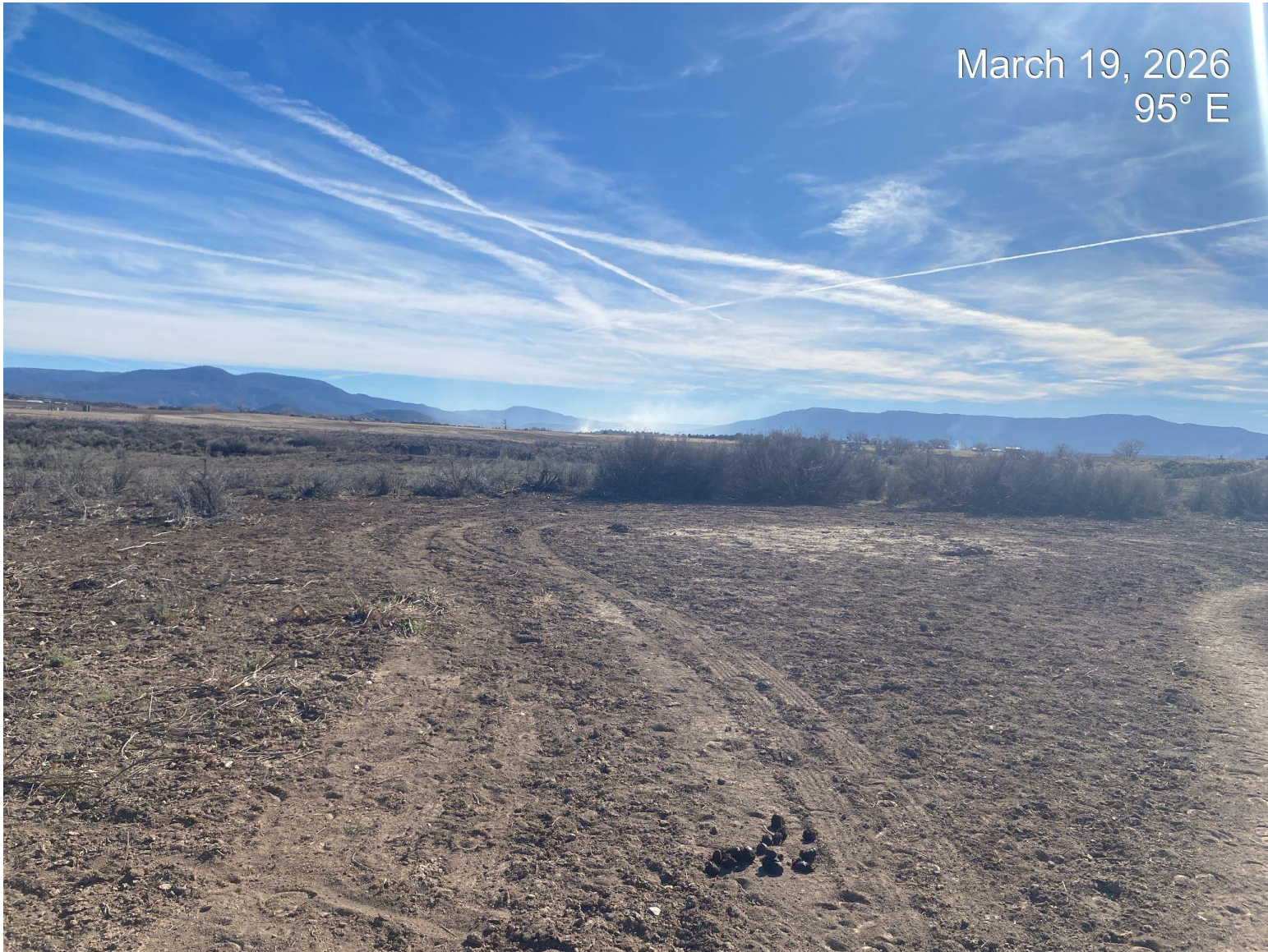
Photo 2. View of the pad portion of the project area taken from the western edge facing center. Note: surface equipment has been removed.
