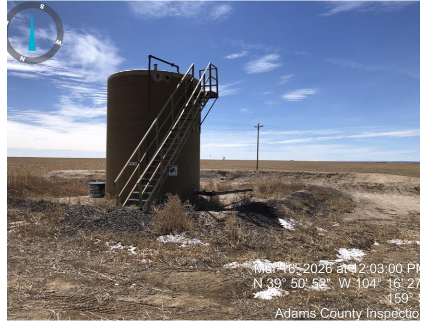
Photo #4 P/W tank.
