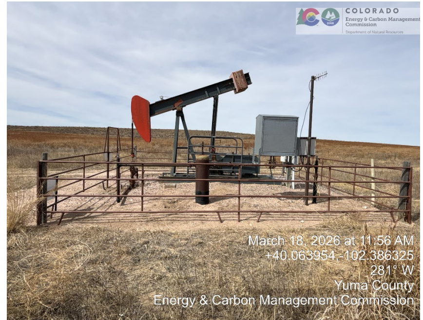
Wellhead, PU, and Meter run
