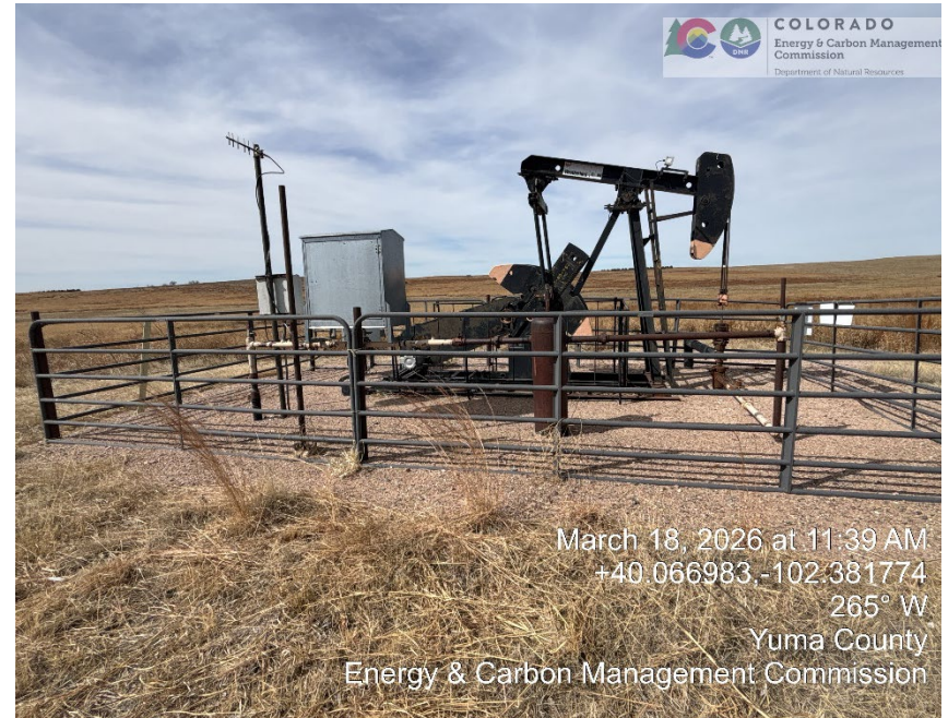
Meter run, PU, and Wellhead
