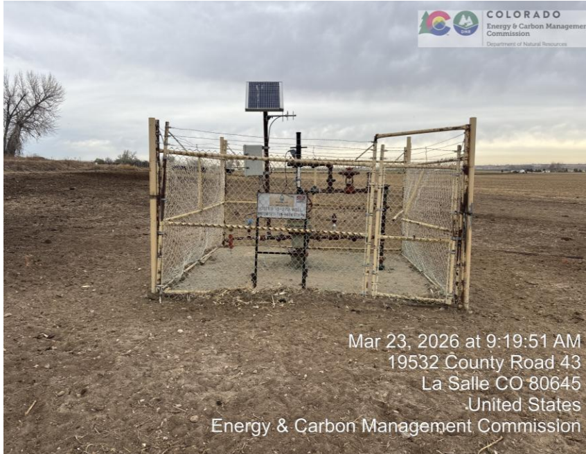
Photo 1 well head and equipment
