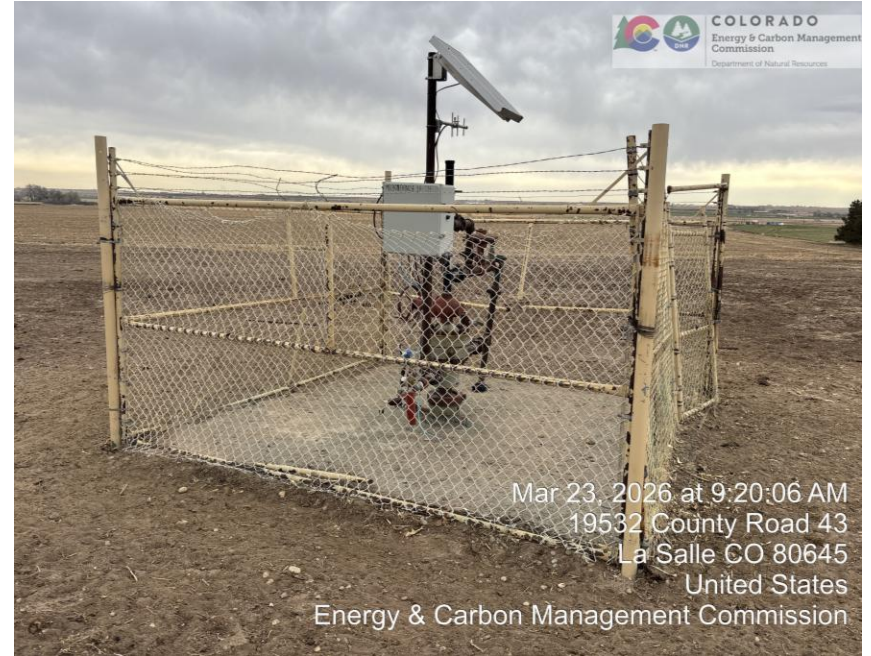
Photo 2 well head and equipment
