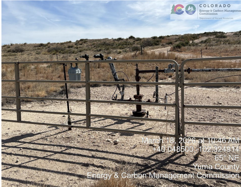
Wellhead and Bellows meter
