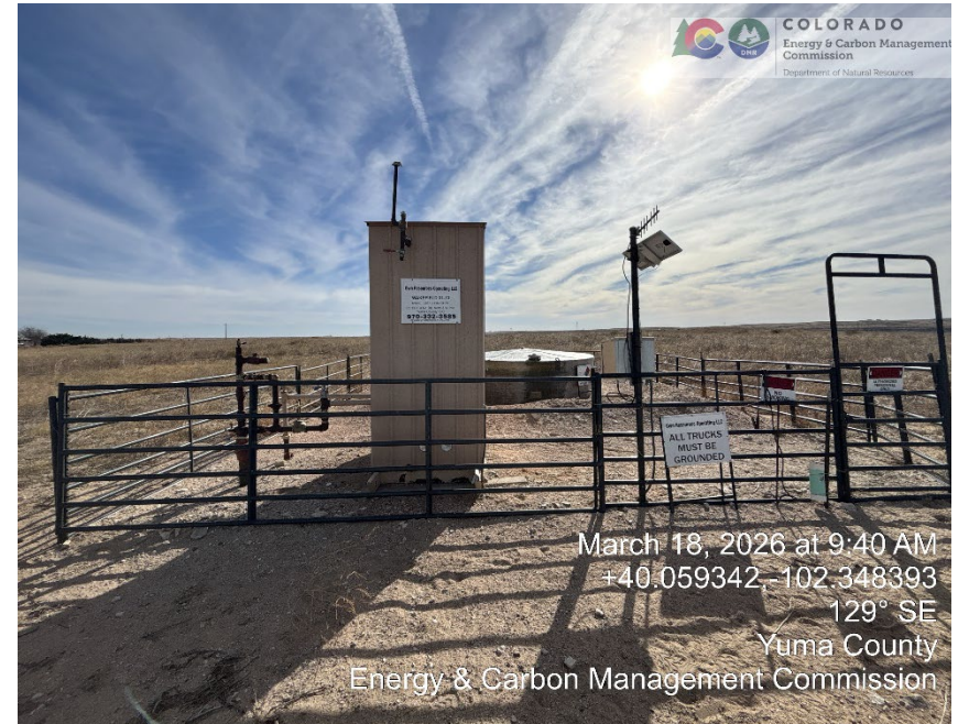
Wellhead and Meter run
