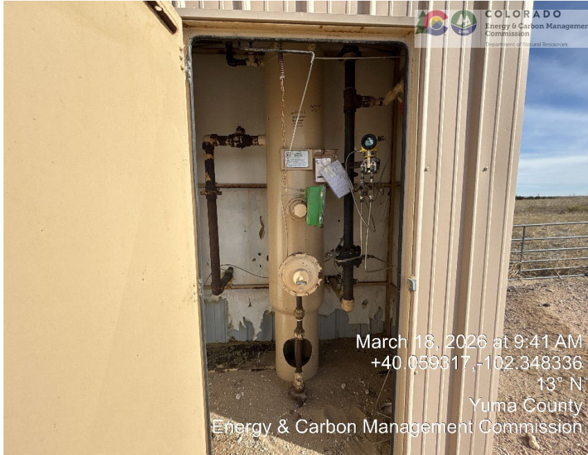
VGS and Meter
