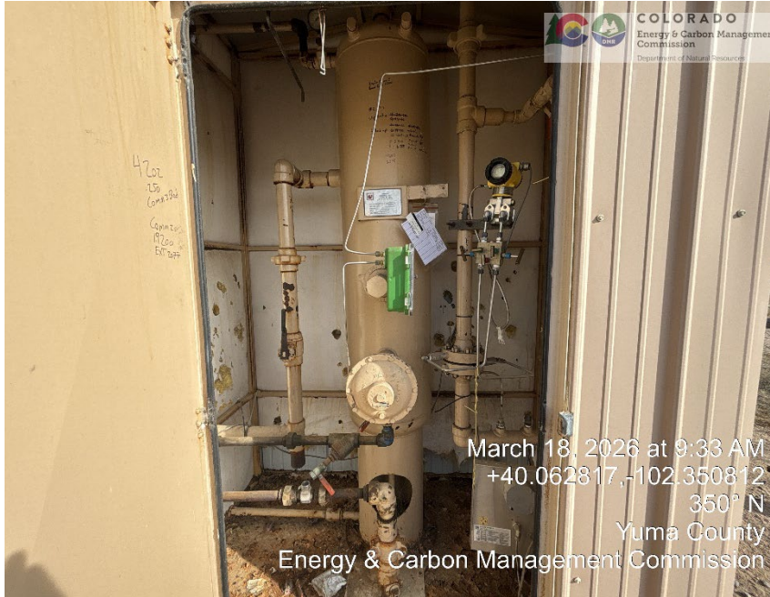
VGS and Meter
