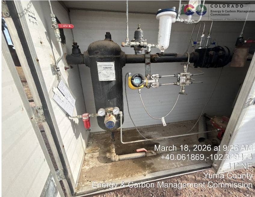
VGS and Meter
