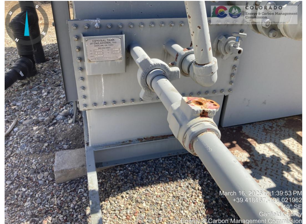
Stem broken off of valve.
