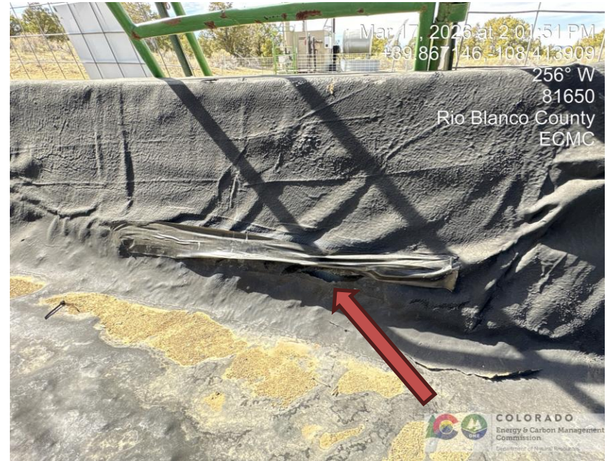
Photo # 3261 Hole in secondary containment liner/liner needs maintenance
