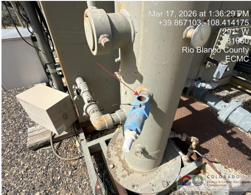
Photo # 3242 PRV vent line does not comply with CECMC pressure safety device rules
