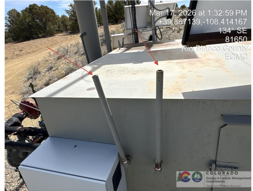
Photo # 3240 PRV vent line & Rupture disc vent line does not comply with CECMC pressure safety device rules
