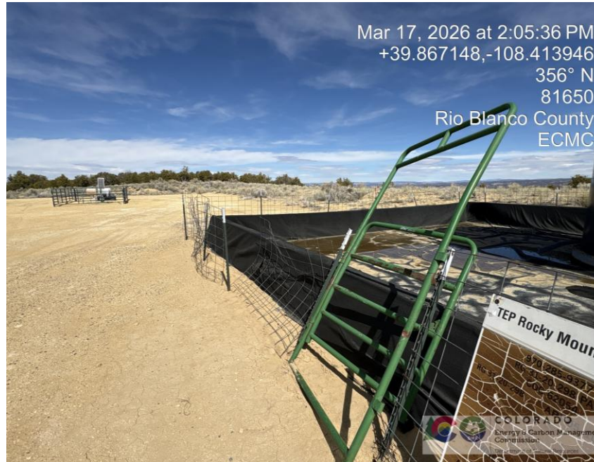
Photo # 3264 Tank battery fencing is in disrepair
