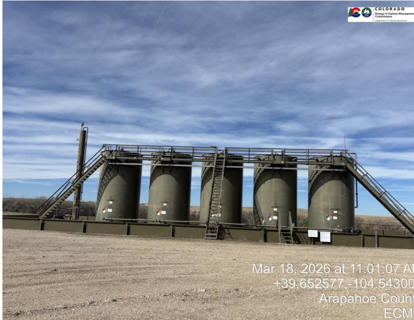
Pic 3 Tanks, VRT
