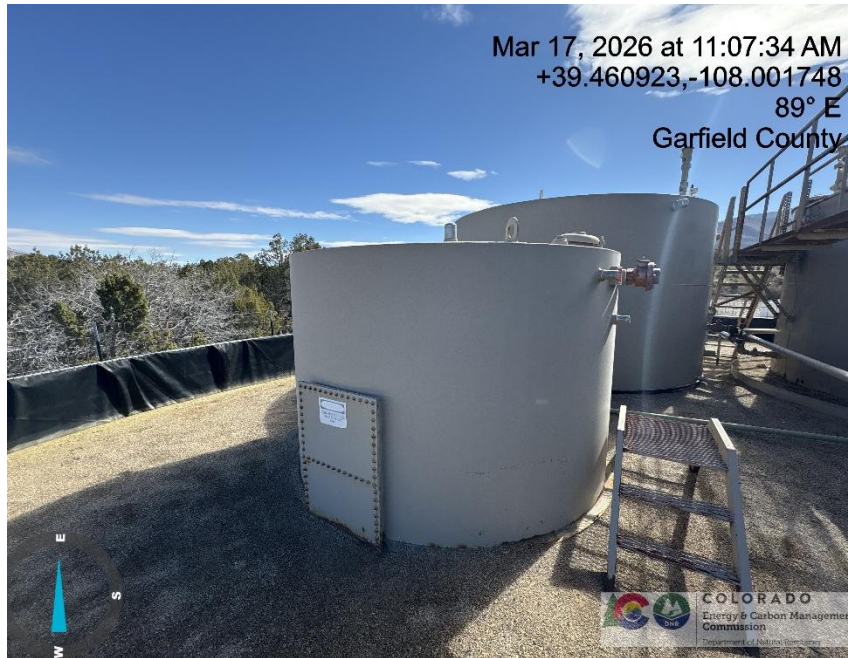
Photo # 9599 Tank disconnected & not in use/unused equipment
