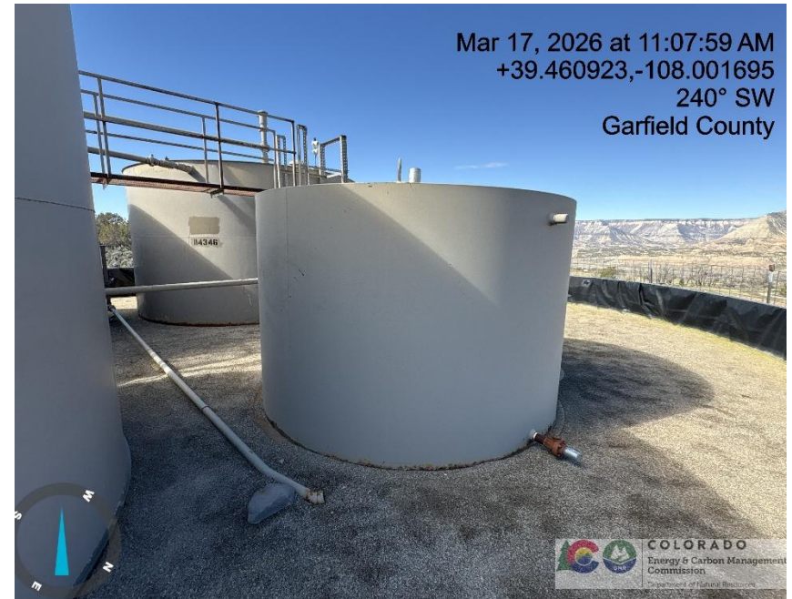
Photo # 9598 Tank disconnected & not in use/unused equipment
