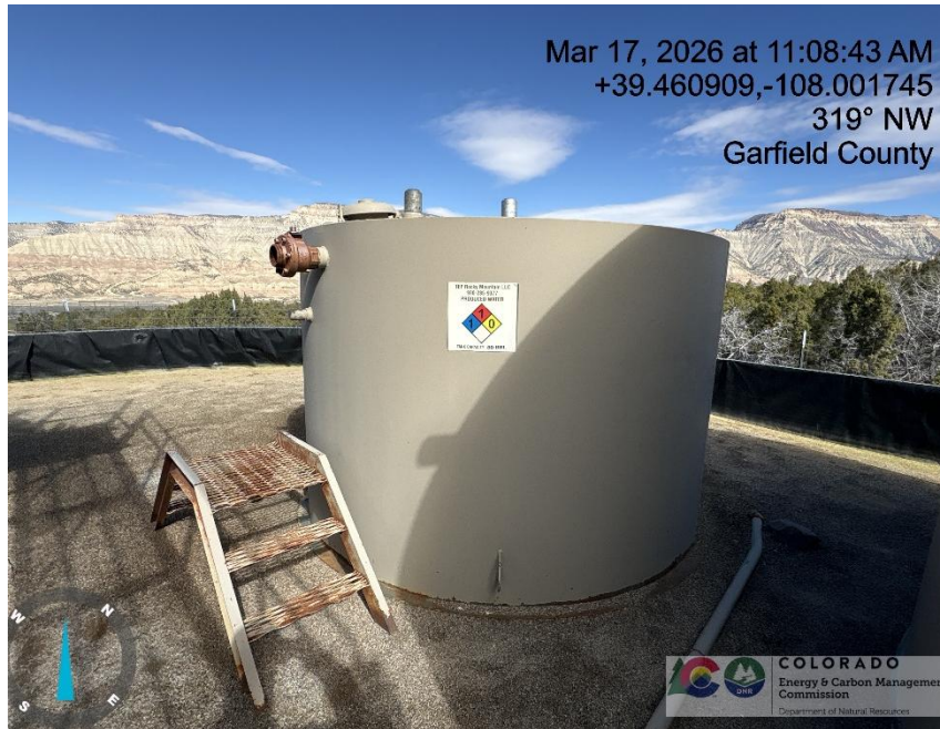
Photo # 9597 Tank disconnected & not in use/unused equipment
