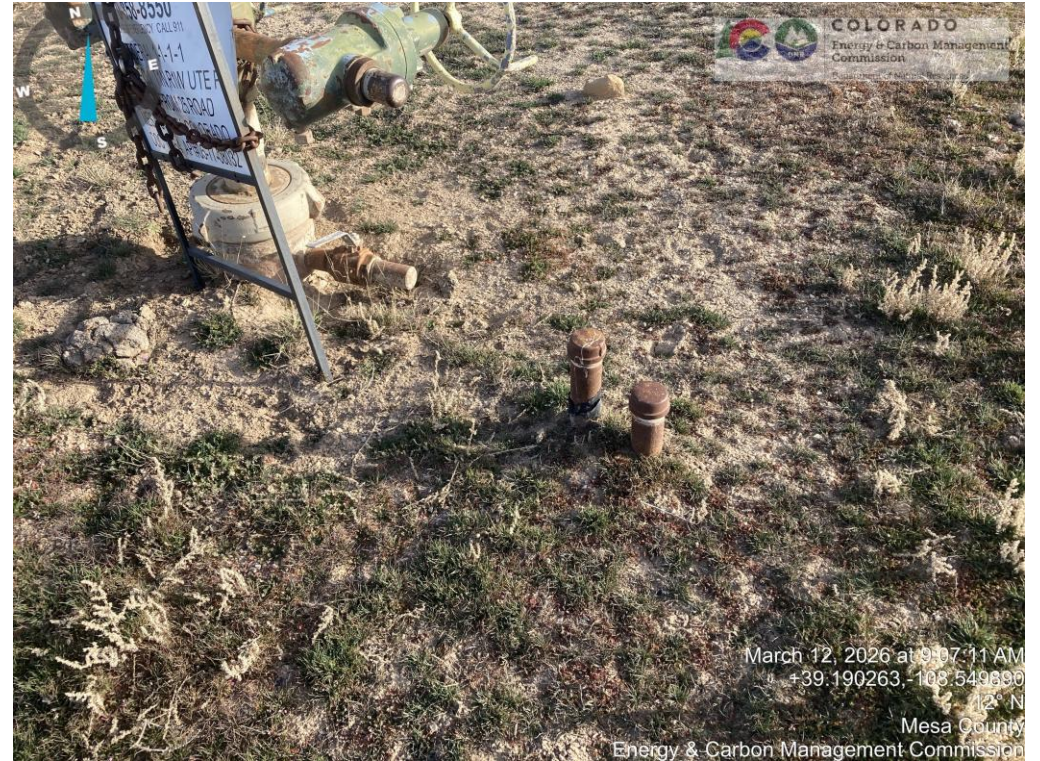
2 flowline risers capped at well head without OOSLAT tags.
