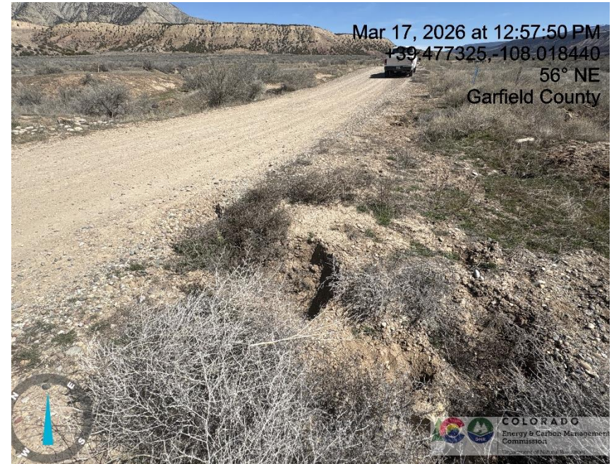
Photo # 9992 Subsidence developing along edge of lease road approximately 1/10 th of a mile from entrance to location
