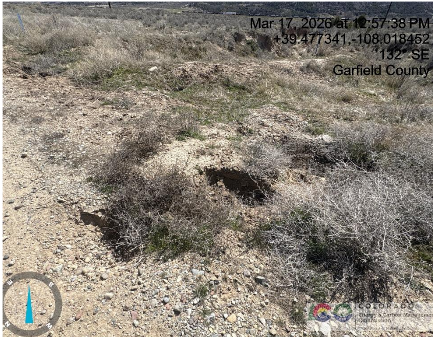
Photo # 9991 Subsidence developing along edge of lease road approximately 1/10 th of a mile from entrance to location
