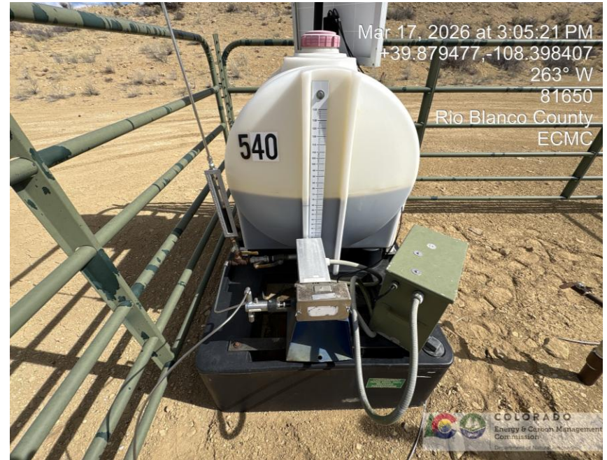
Photo # 3301 Failure to maintain chemical BMP/chemical containment approximately 3/4th full of fluid/not sufficient to contain possible spill
