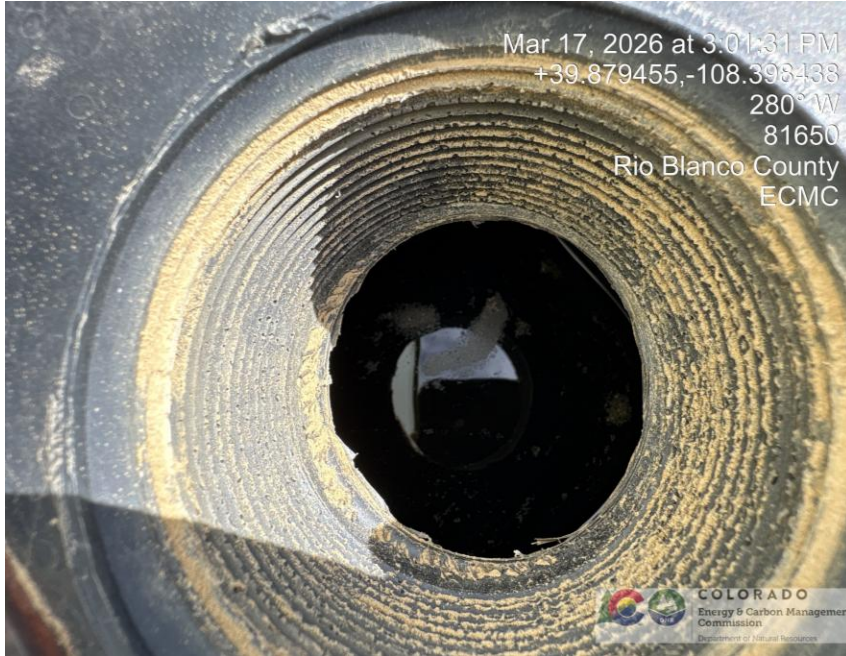
Photo # 3297 Failure to maintain chemical BMP/chemical containment approximately 3/4th full of fluid/not sufficient to contain possible spill
