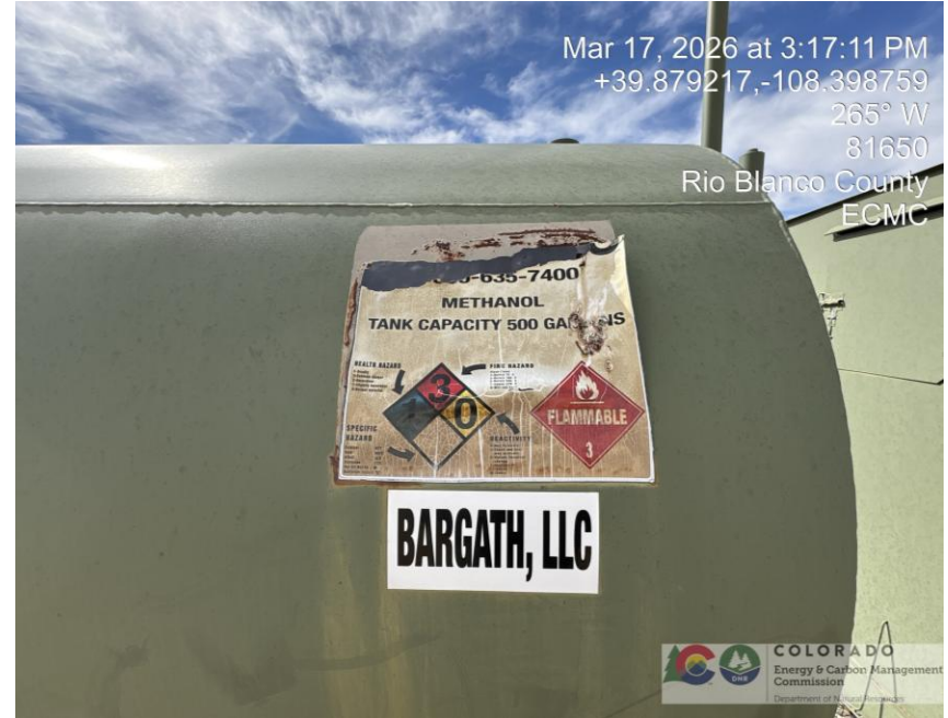
Photo # 3311 Methanol tank label is damaged/weathered, lacks required information
