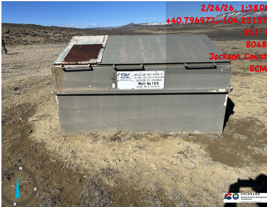
Well head signage
