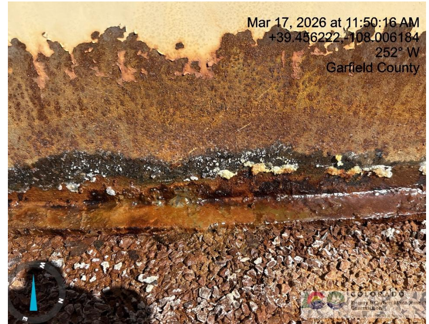
Photo # 9768 Tank failure/Tank lacks integrity
