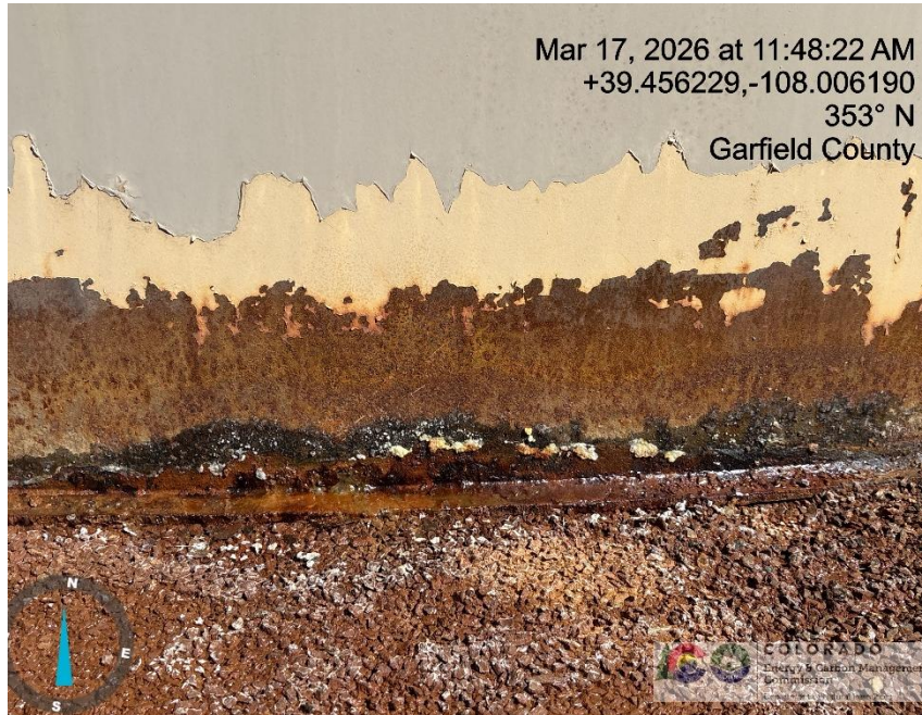
Photo # 9767 Tank failure/Tank lacks integrity
