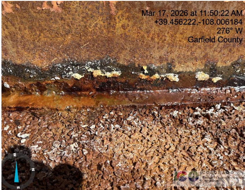
Photo # 9769 Tank failure/Tank lacks integrity
