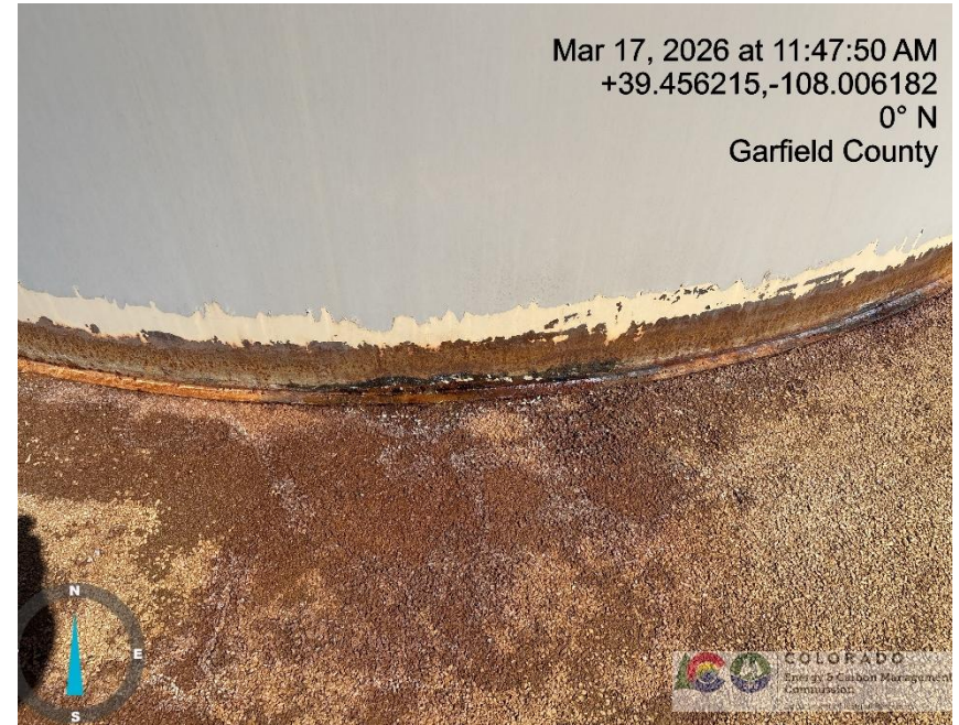
Photo # 9764 Tank failure/Tank lacks integrity
