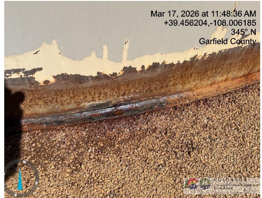
Photo # 9770 Tank failure/Tank lacks integrity
