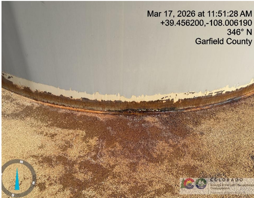
Photo # 9763 Tank failure/Tank lacks integrity
