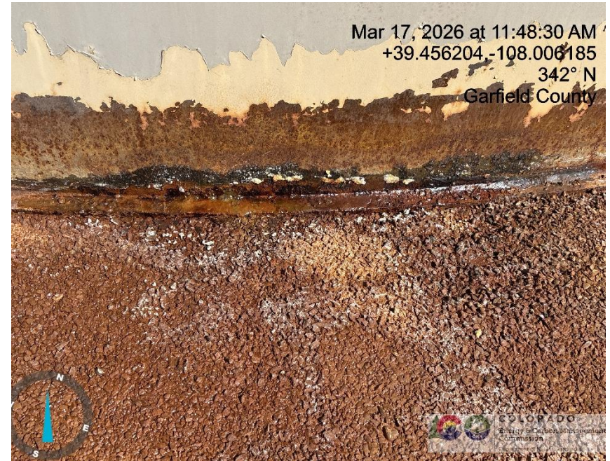
Photo # 9766 Tank failure/Tank lacks integrity
