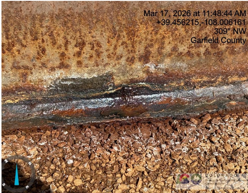
Photo # 9771 Tank failure/Tank lacks integrity
