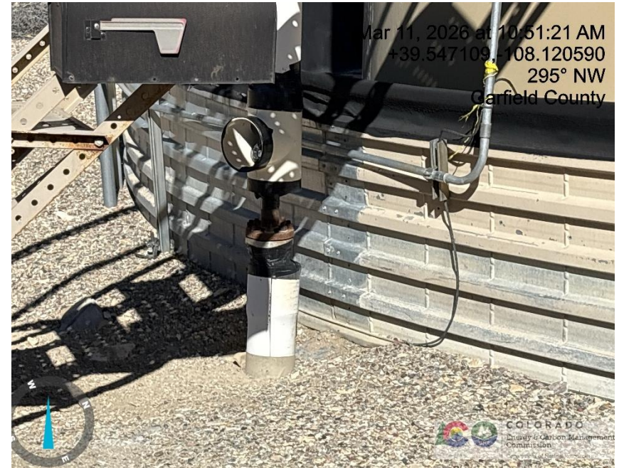
Photo # 8377 Flowline heating insulation open ended /wildlife hazard/available for entry by wildlife
