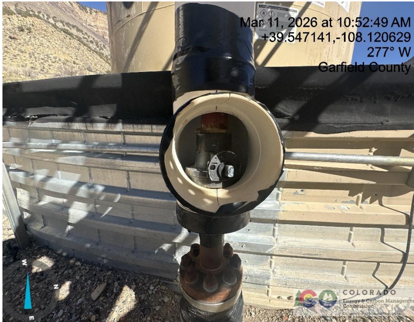
Photo # 8378 Flowline heating insulation open ended /wildlife hazard/available for entry by wildlife
