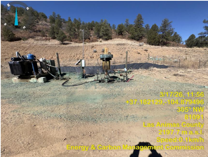
Photo 9 Wellhead Gas Skid engine.
