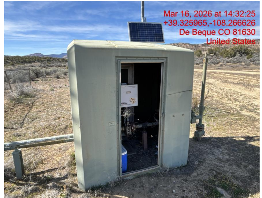
Unsecured Gas Meter House – Photo #03109
