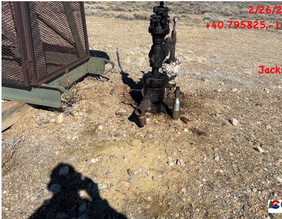
Staining and open line
