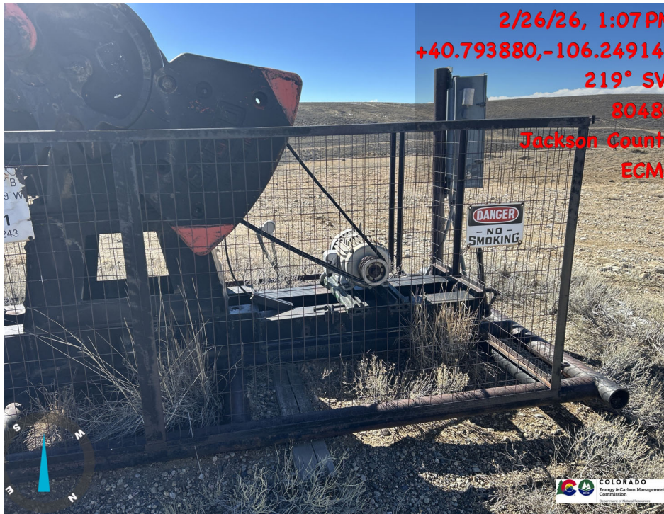
Belt guard missing
