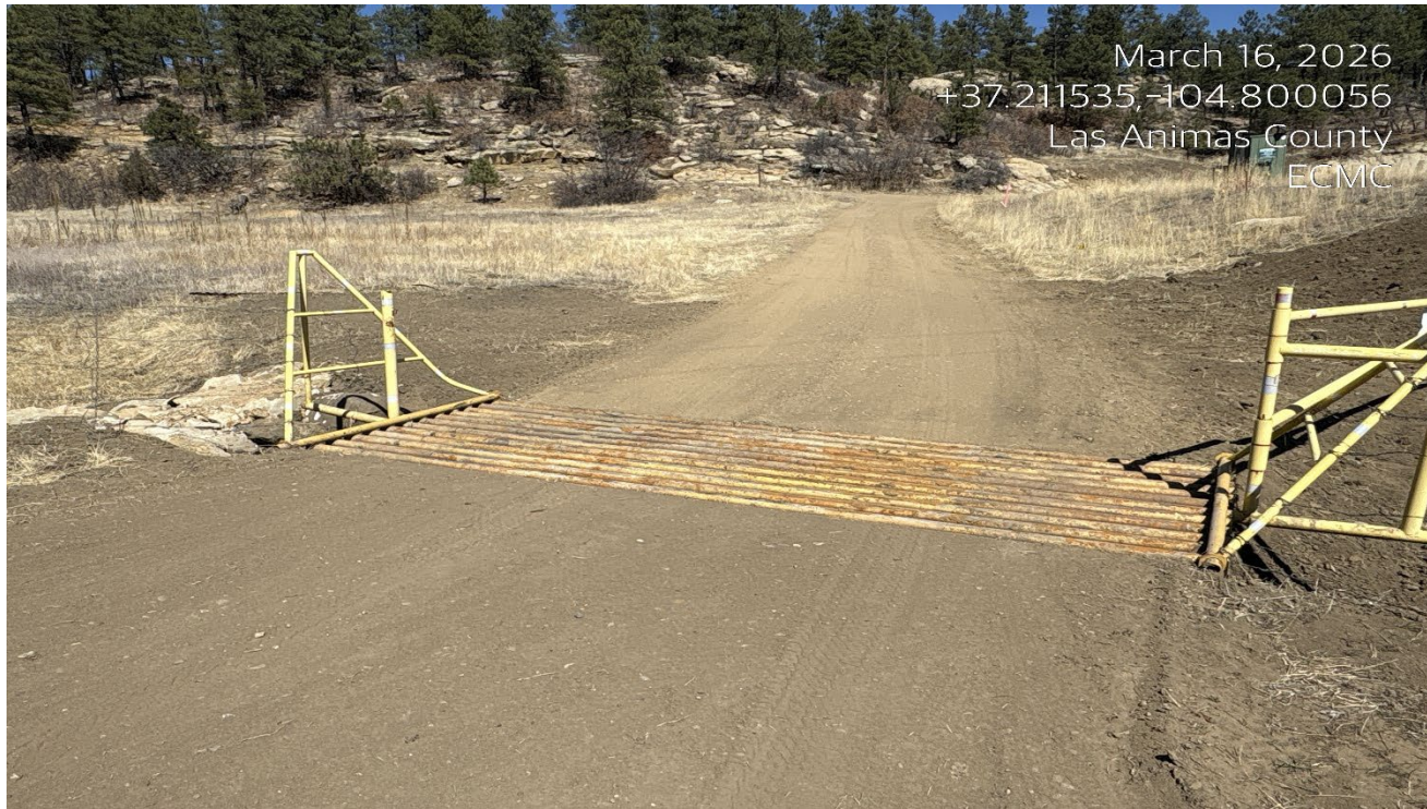
Photo 1. Facing northeast at the access road. The cattle guard has been cleaned out and is in good condition.
