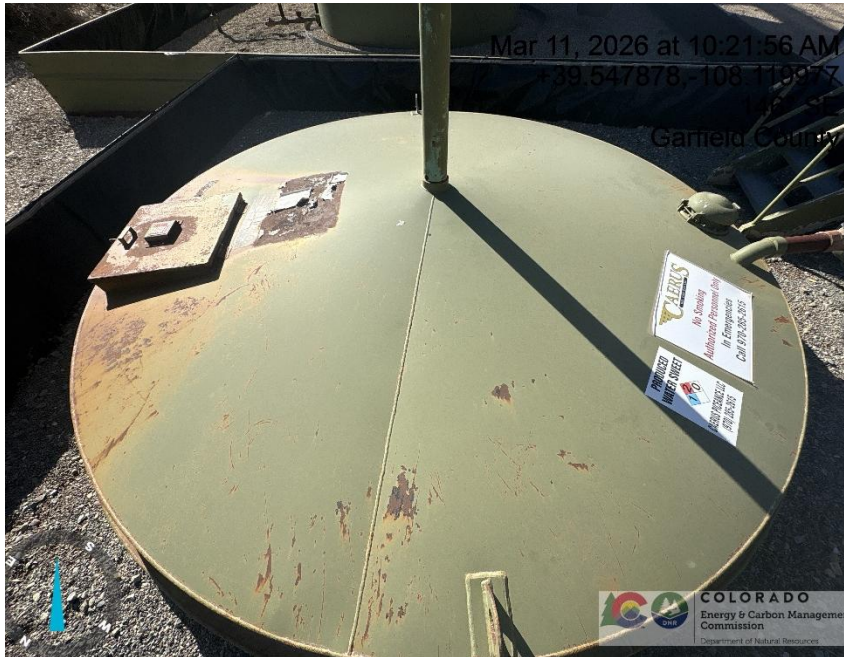
Photo # 8216 Partially buried tank lacks capacity – additionally tank labels have previous operator name
