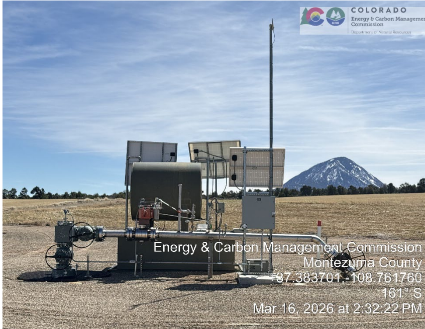
7. Wellhead, stainless flowline, 1000 gallon produced water/diethylene glycol tank atop secondary containment tank with expanded metal screen, and solar telemetry. Plowed agricultural field surrounding pad.
