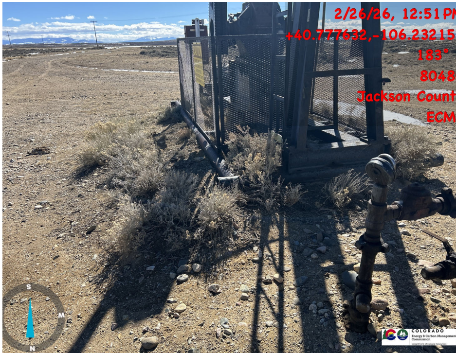
Weeds around equipment
