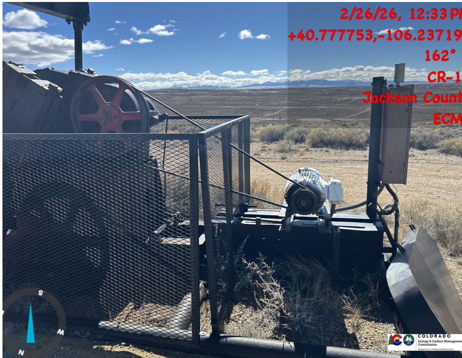
Missing belt guard
