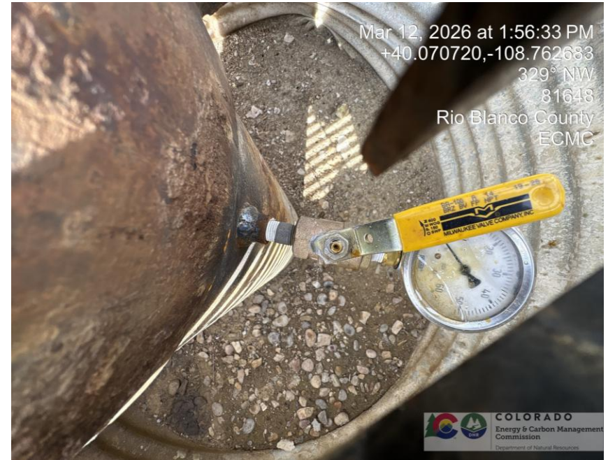
Photo # 3018 Bradenhead valve is accessible/equipped with gauge
