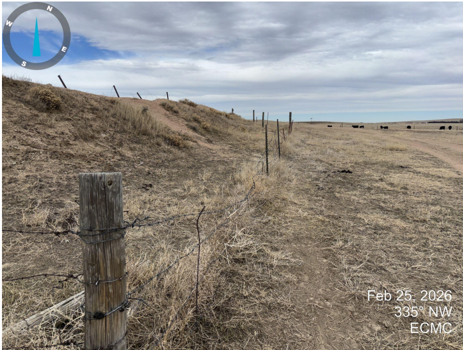
Photo 9. Looking north along the east side of the south pit. Desirable vegetation is present in this area. Fence is loose and down around both pits. Debris including netting and metal scrap is present around the pits.
