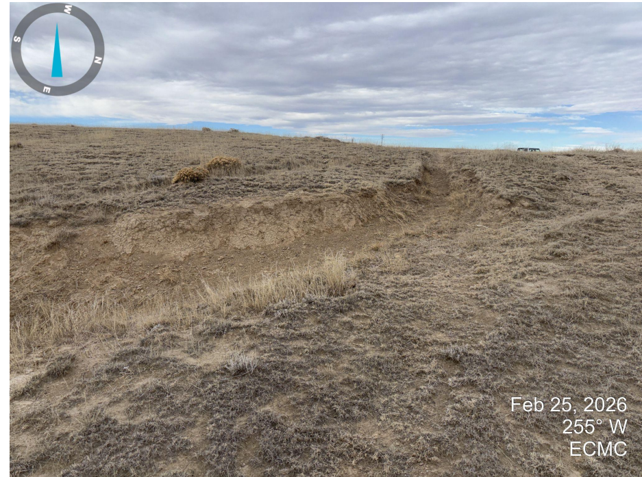
Photo 8. Closeup photo of erosion channel from the tank battery pad. Channel forms at the southeast corner of the tank battery pad and gully erosion is present. Livestock may be contributing to erosion.
