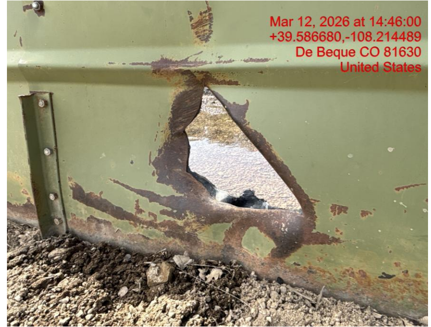
Punctured Berm Wall – Photo #03058
