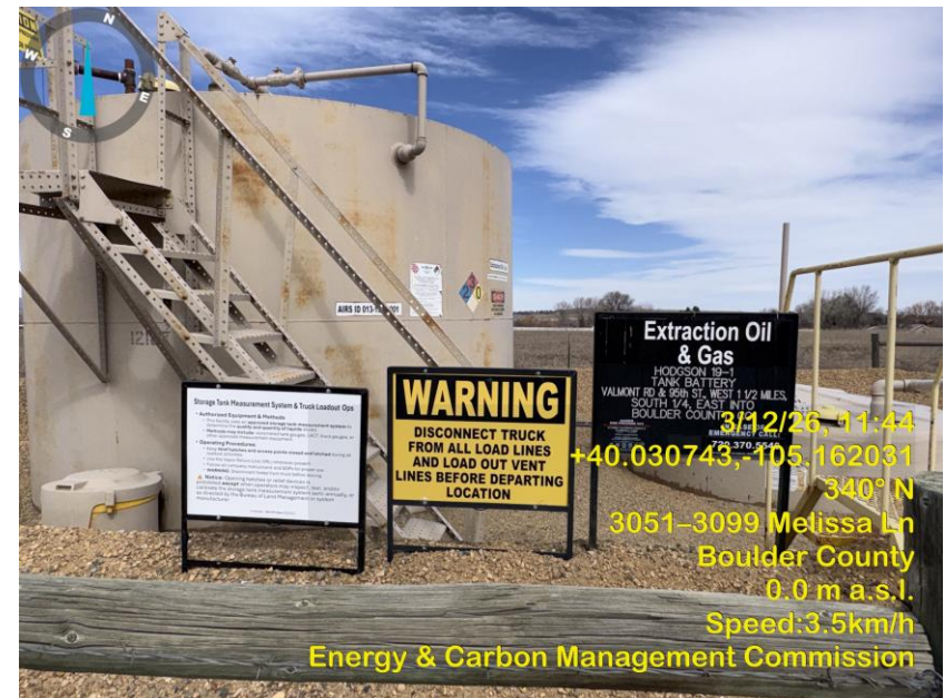
Photo 4 Tank battery signs.
