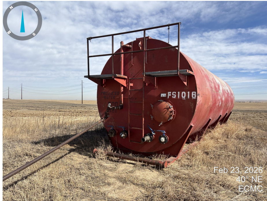
Photo 5. Produced water tank with no secondary containment.
