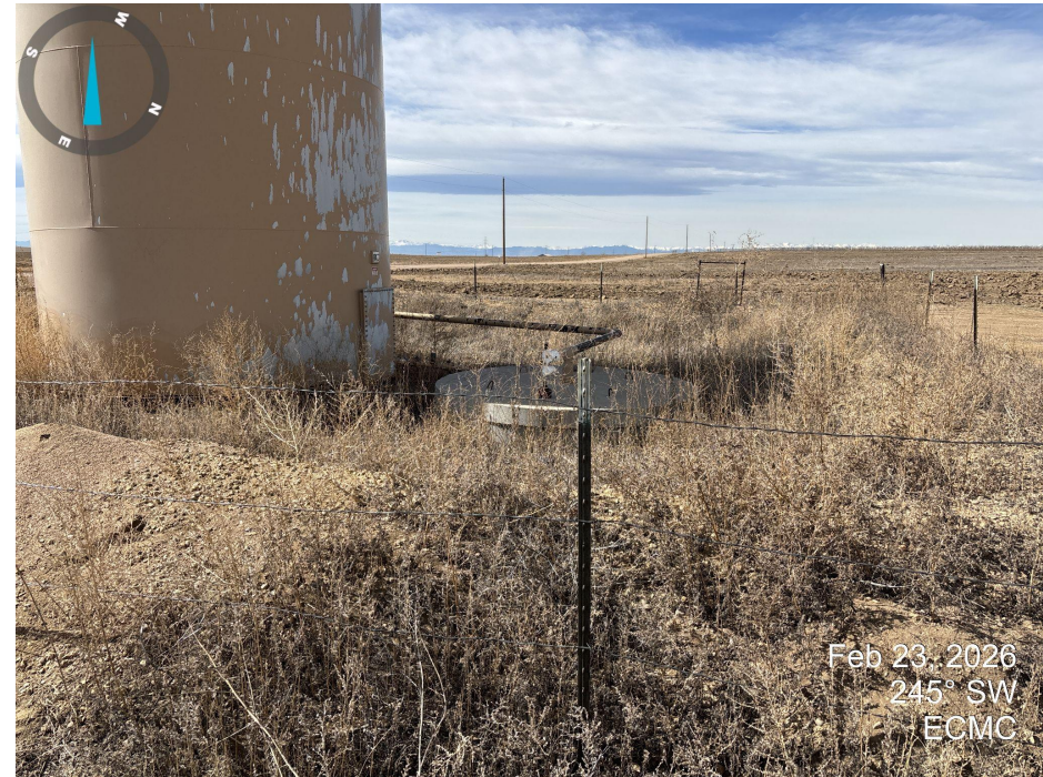
Photo 2. Looking west across tank battery. Weeds present inside secondary containment.
