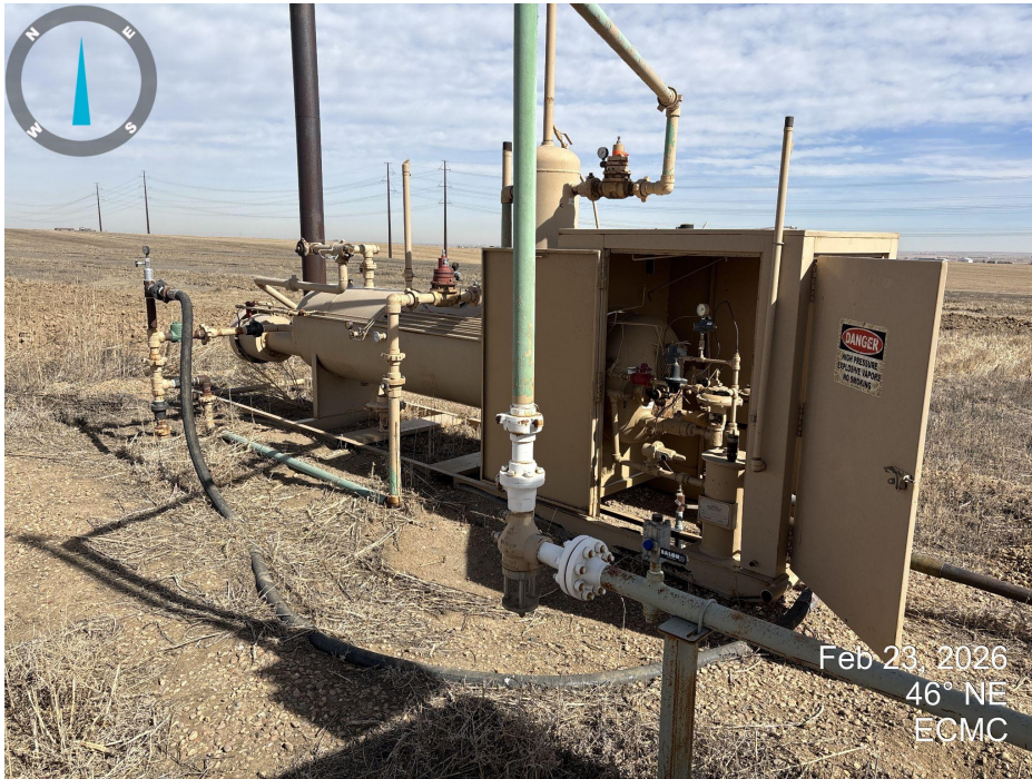
Photo 3. Separator on location.
