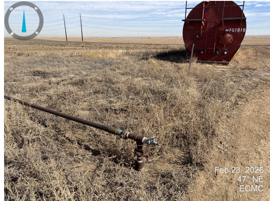
Photo 4. Looking northeast near the separator and produced water tank. Produced water tank does not have secondary containment.
