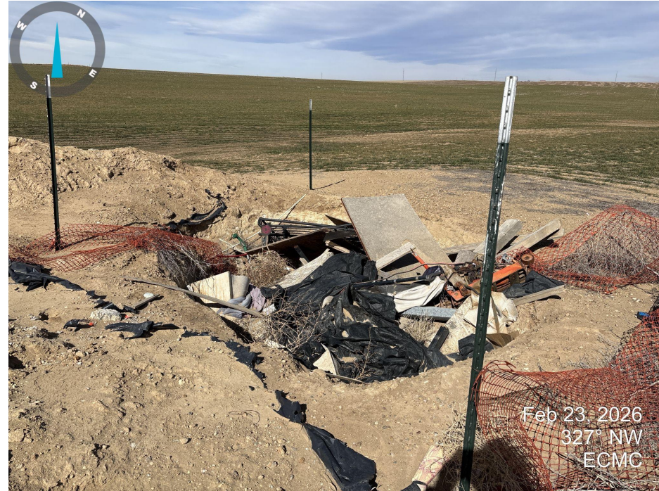
Photo 4. Looking north across the open excavation and wellhead. Trash and debris is present in the open excavation.
