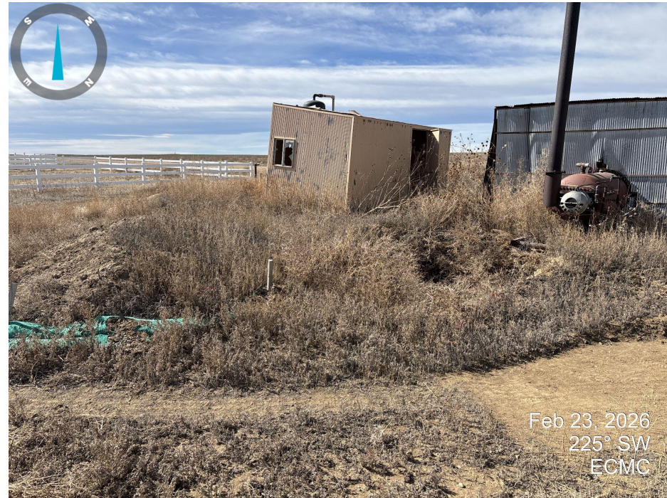
Photo 4. Looking south at the separator sheds on the southern side of location. Excavation and soil pile appear unchanged since last reclamation inspection (04/15/2025).
