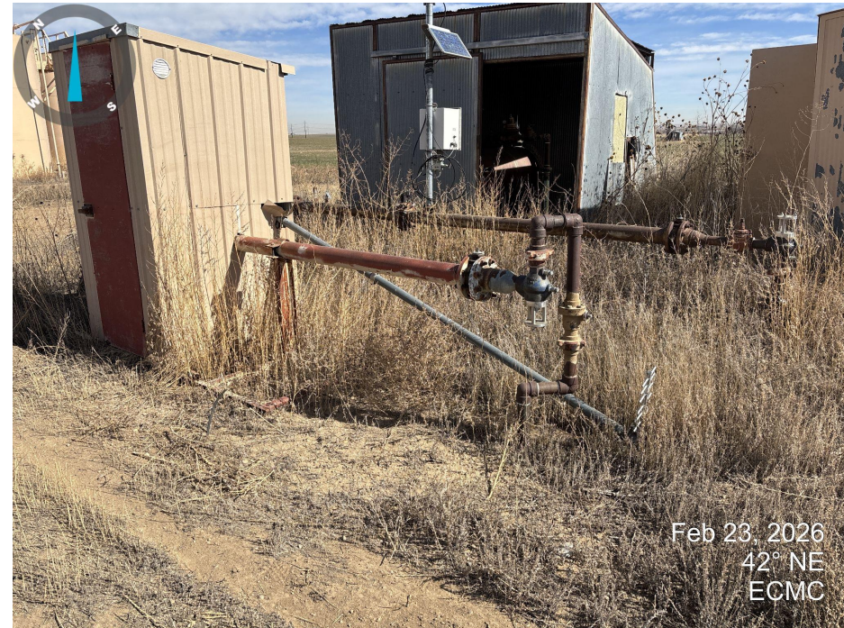
Photo 6. Looking east across the separator sheds. Weeds are present throughout the location.
