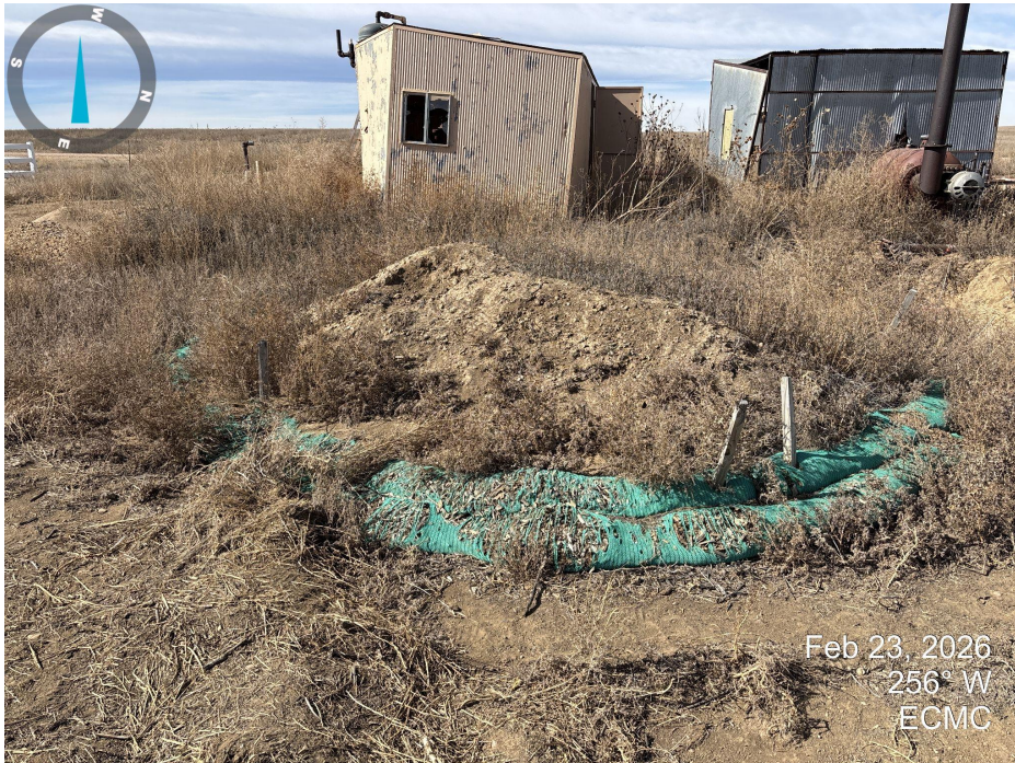
Photo 5. Soil pile remains on location. Stormwater BMPs around soil pile have degraded.
