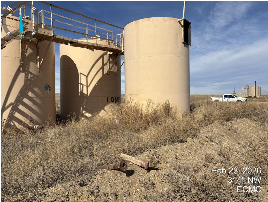
Photo 3. Looking northwest at the east side of the tank battery. Undesirable weeds inside of secondary containment. Unused equipment remains on site. The eastern tank has an open inspection hatch.
