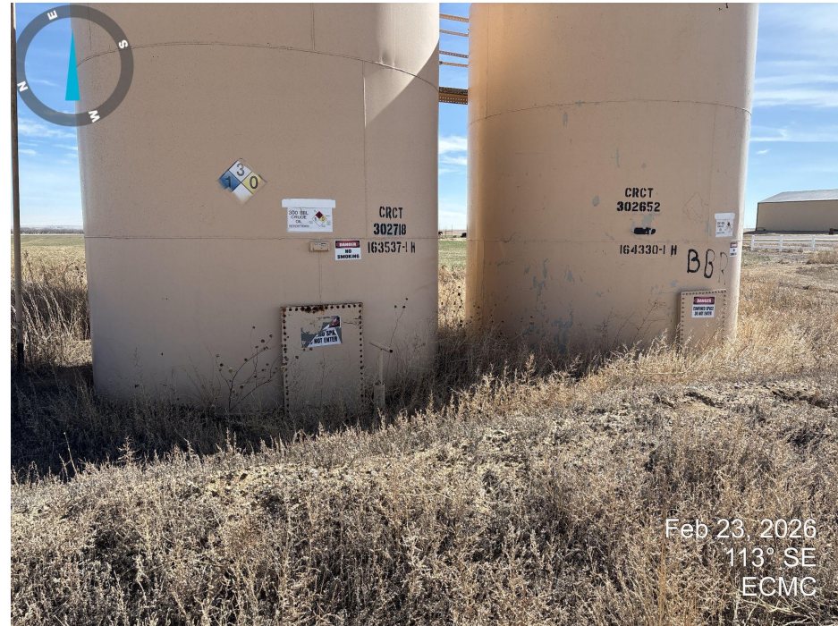
Photo 2. Looking east across the tank battery area. Undesirable weeds such as Kochia and Russian Thistle are present inside of secondary containment.
