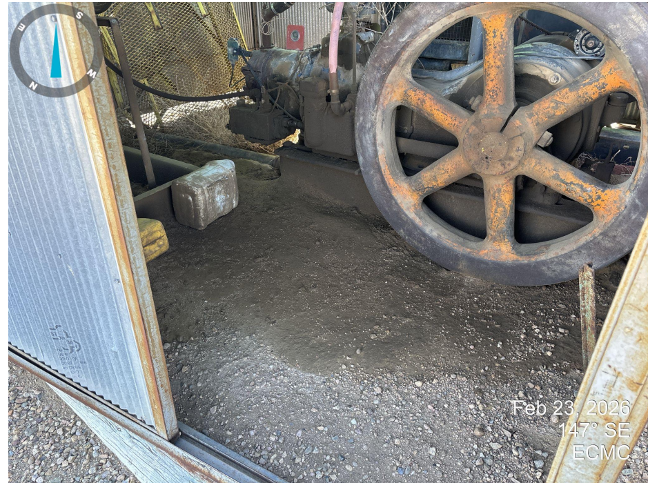
Photo 4. Stained soil present around engine. Close engine shed door to prevent unauthorized access. Flywheel does not have cover installed.
