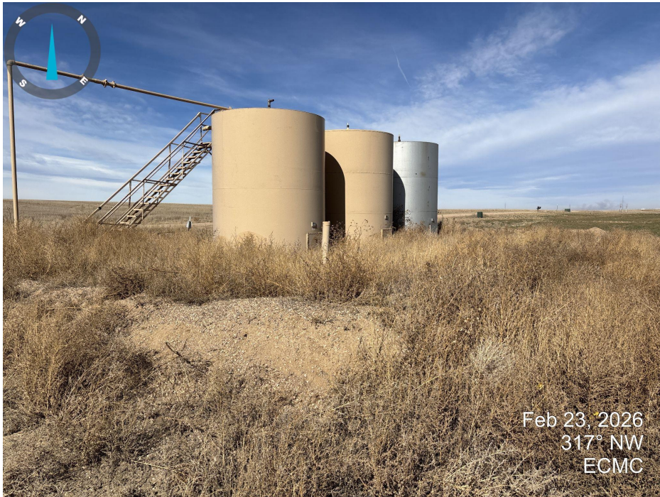
Photo 7. Looking northwest across tank battery. Weedy undesirable plant species were present and unmanaged throughout location (Kochia, Russian thistle).
