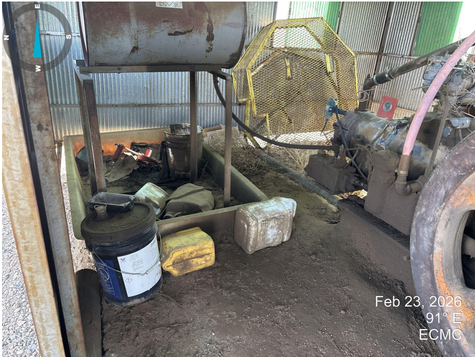
Photo 3. Trash and debris is present inside the motor shed.
