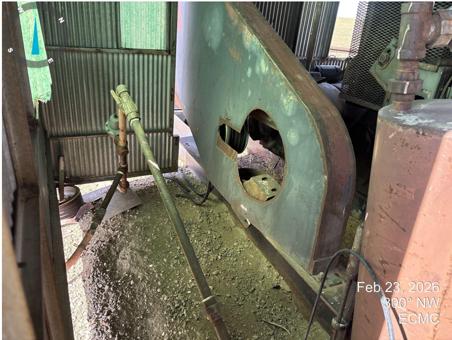
Photo 5. Broken belts left in place around pulley.
