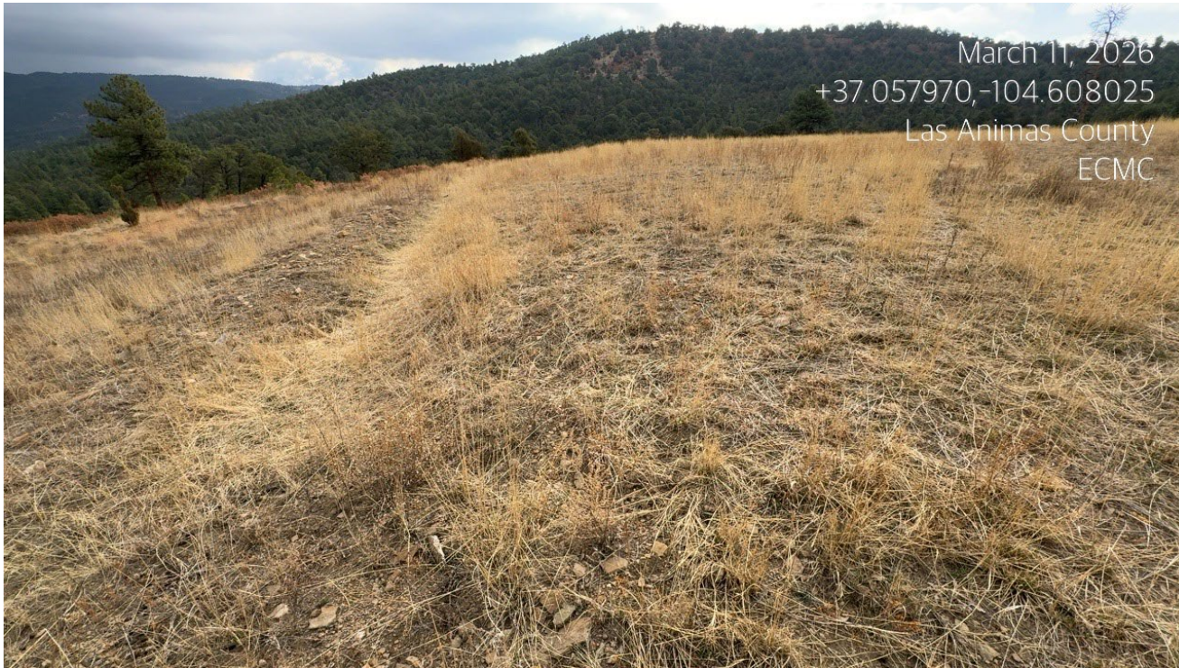
Photo 6. Facing east along the fill slope of the location which is stabilized with perennial desirable vegetation.
