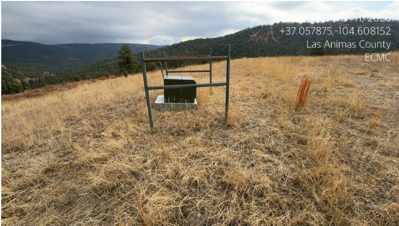
Photo 5. The buried electric utilities remain at the location per approved variance.
